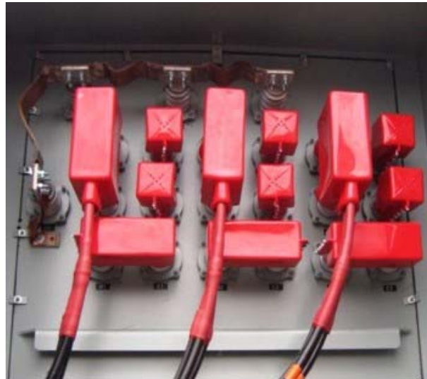
XFMR Bushings on the Installation Date
