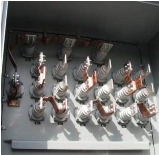
XFMR Bushings on the Measurement Date
